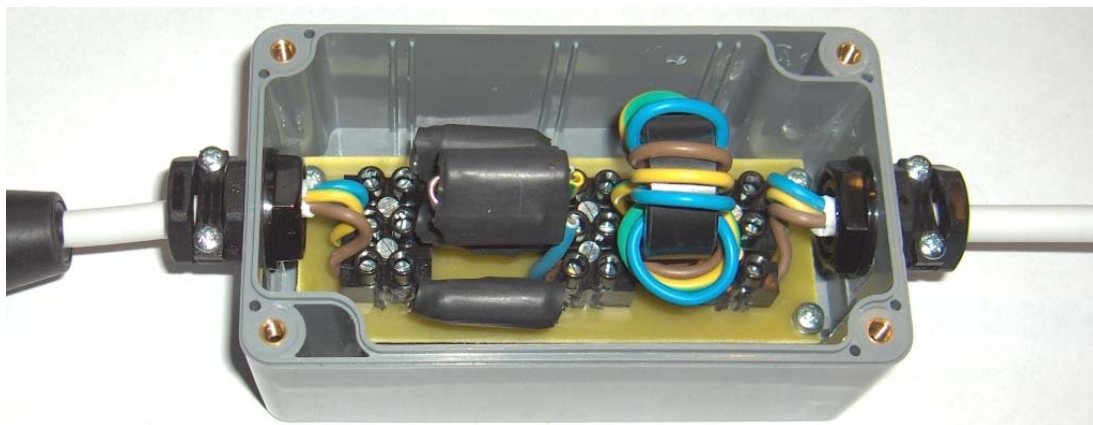
Figure 45: Filter View Inside
